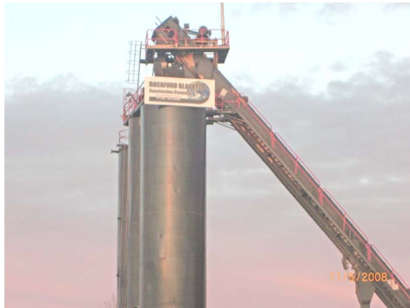
The asphalt silo
