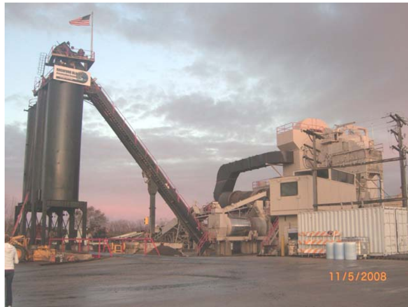
This is the control center, asphalt silos, and barrel furnace
